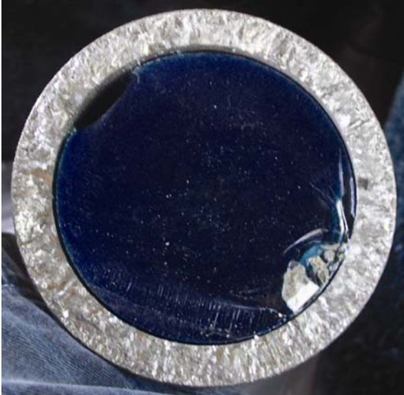
CC PS 413 in 4-inch Dur-Iron pipe
